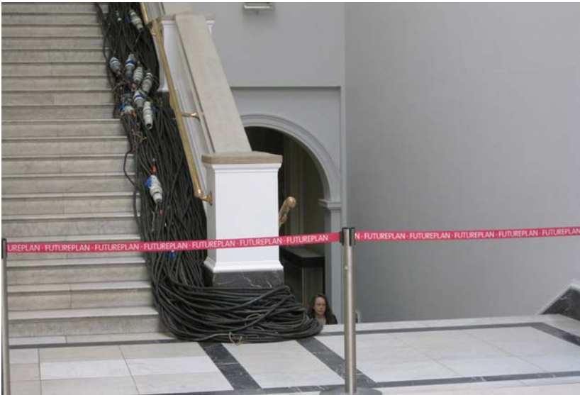
Cabling at the Victoria and Albert Museum, London. One should let experts lay cables for travelling exhibitions to avoid overheating or the risk of people tripping. Photo: Mathias Strömer.
